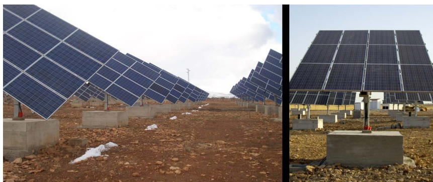
Fig. 2. Detail of the PV plant and the tilted one-axis tracker.
