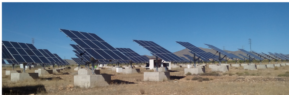
Fig. 1. PV plant under analysis.
