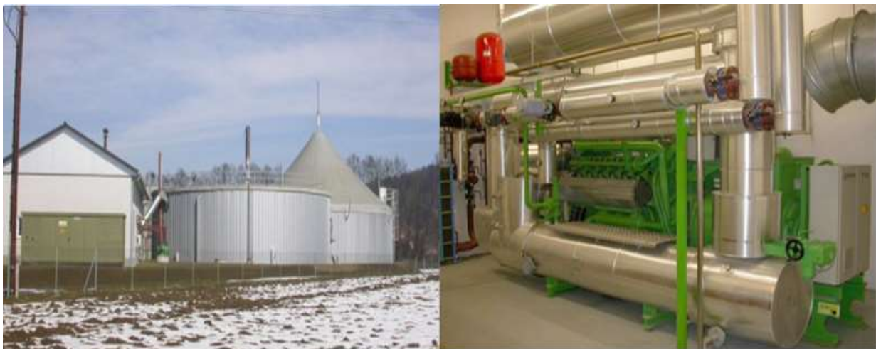
Figure 1-27 A biogas facility employing the anaerobic digestion of manure (on the left) in conjunction with a Jenbacher® gas engine (on the right).
