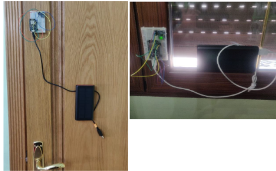
Fig. 3: Device installed on the door and window.
